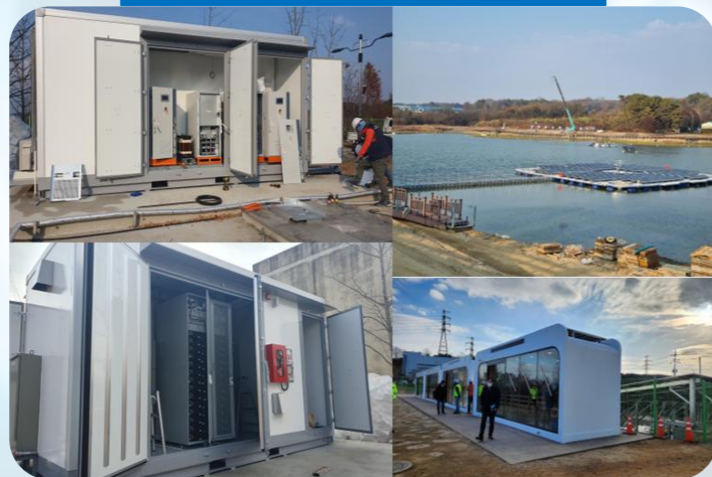
PV + BAT Off-grid DC-ESS (진천)
