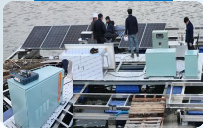
On Water Off-grid Hybrid ESS (옥천)
